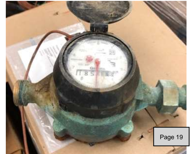
Failing Water Meter
